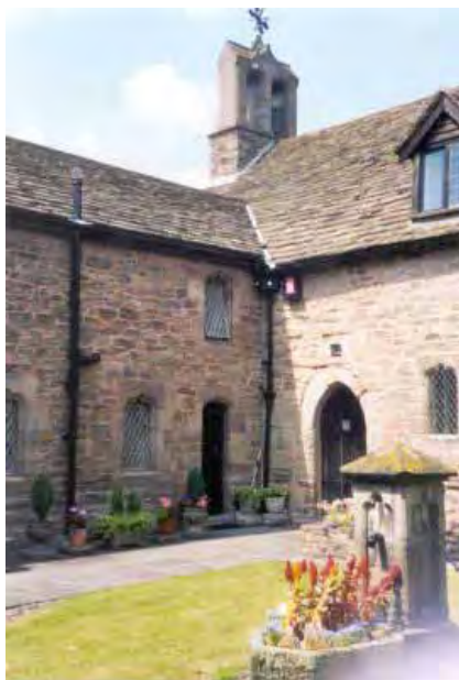
Figure 13. Courtyard of the Coningsby Hospital. The size grading on the stone tiles on the roof, small at the ridge and bigger towards the eaves is well seen
