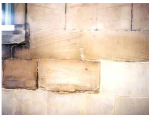
Figure 31. Close-up of the cross-bedded sandstone ashlar blocks fronting the Shire Hall. Open cracks show the need for further restoration.
