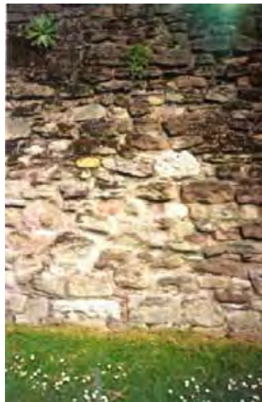
Figure 6. Close-up view of the roughly shaped stonework of the city walls. Local Old red Sandstone is mainly used, but other lithologies were also used, for example the white and yellow blocks in the centre of the picture
