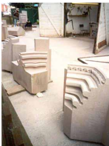
Figure 61. The Mason's Yard in front of the North Transept, showing replacement masonry.
