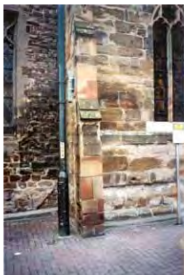
Figure 7. Stone work near the south doorway of All Saints Church, in roughly shaped Old Red Sandstone, the mediaeval walling being patched with ashlar blocks of Triassic Hollington Stone from Staffordshire
