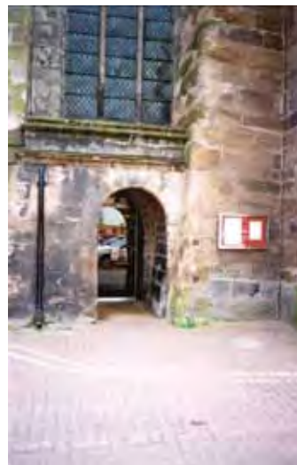
Figure 8. Romanesque north doorway of All Saints Church, in roughly shaped "old red sandstone" blocks
