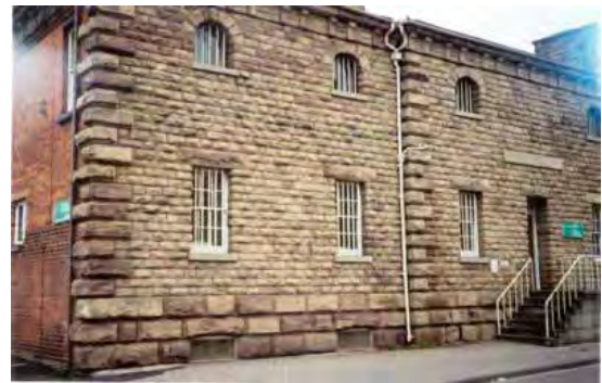
Figure 29. Rusticated façade of the Gaol and Police Station in Gaol Street: note the brick construction of the remainder of the building.
