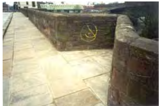
Figure 3. Showing the weathered sandstone of the bridge walls and the new sandstone paving
